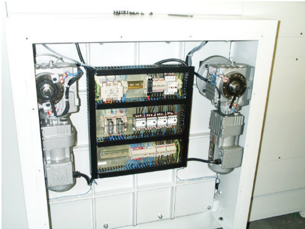
Fig. 3 Inner Door Control Panel at Rear
