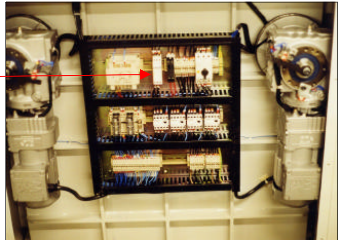
Rear Inner Door Control panel showing Phase Rotation Detector Unit
