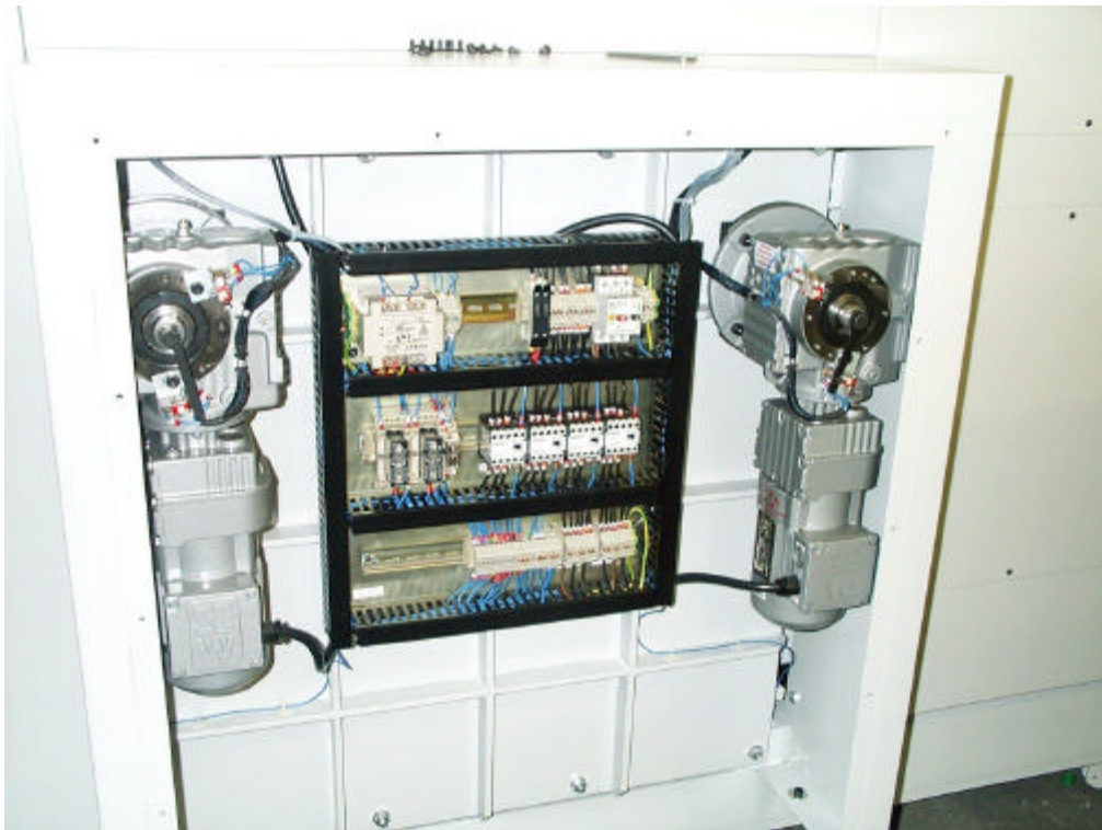
Fig. 3 Inner Door Control Panel at Rear
